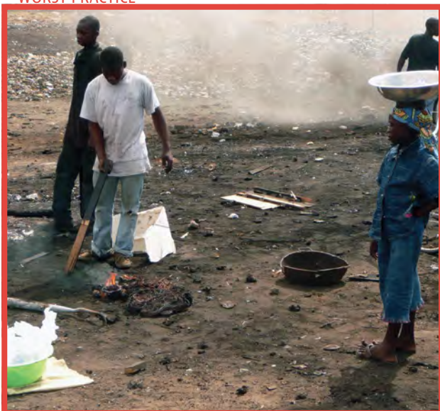
Ghanaian boy off-burning plastics from copper cables and a girl bringing water, Accra, Ghana ©Empa
